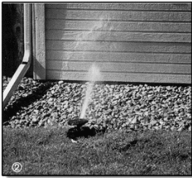
Adjust your sprinkler heads so they water the intended areas and not walls and rocks as shown here.
